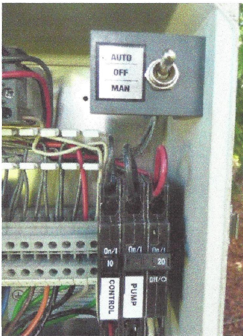
Figure 2 Typical pump controls (top) and circuit breakers (bottom) found inside control box.
