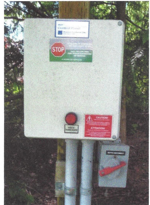
Figure 1 Typical septic tank control box with red indicator button (center) and main power switch (bottom right).
